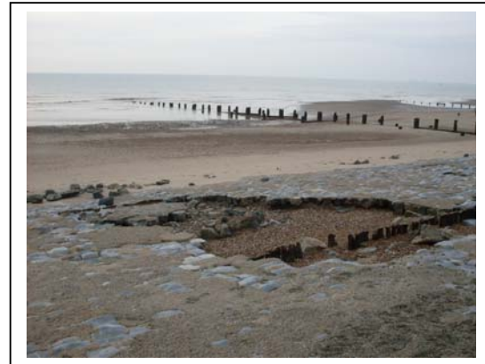
Damage to existing sea defences
