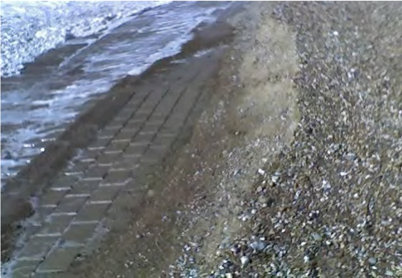
Embankment just crumbling away – 1 hour yet to go for high tide!
