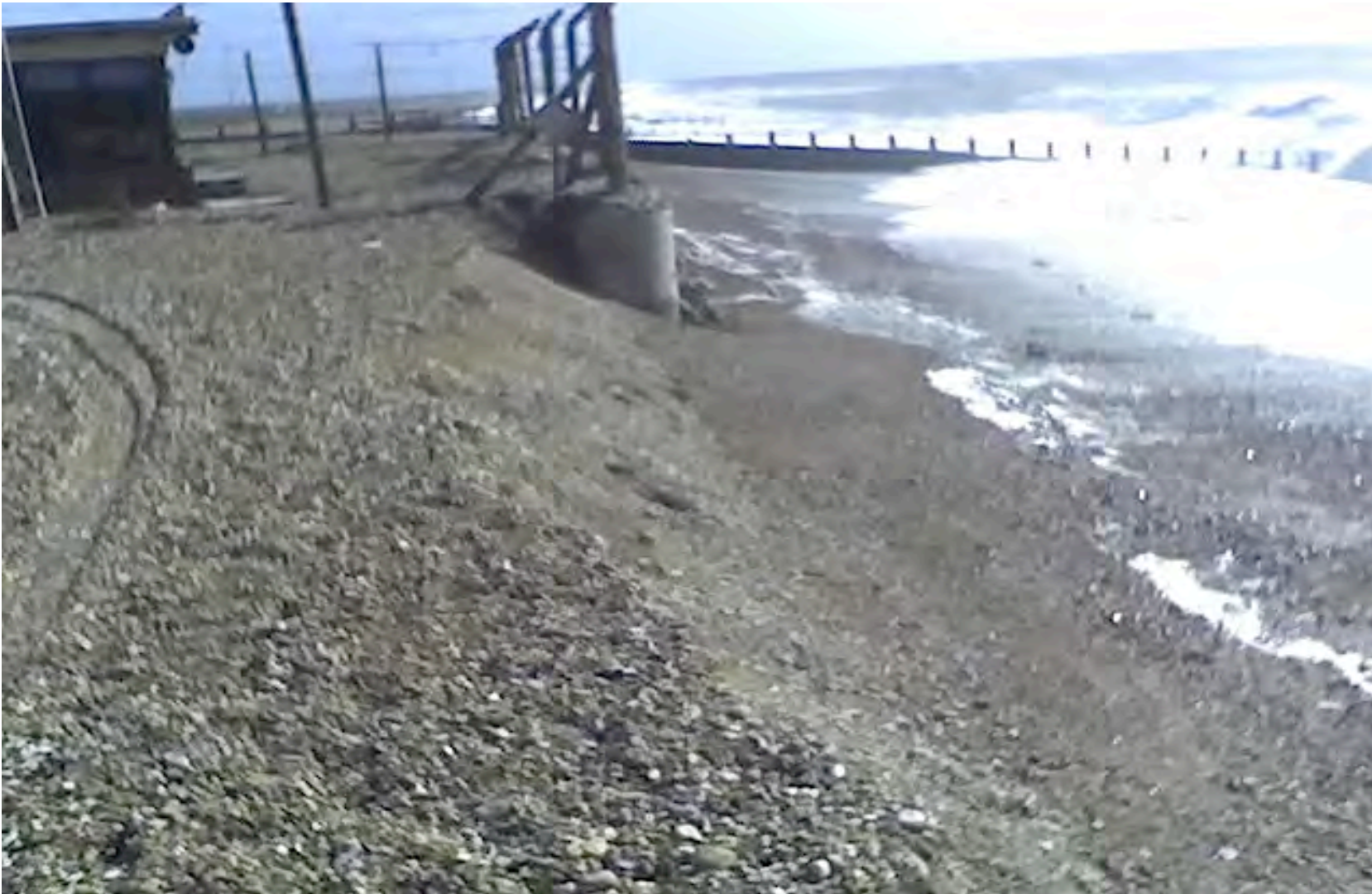
MOD Lookout – all shingle ridges gone – base of structure totally exposed
